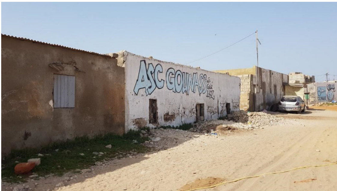
Housing damaged by floods, Médina Gounass, in Guédiawaye (north of Dakar) Photo by Bea Varnai (2019)
